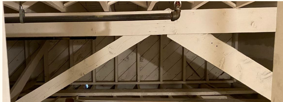
View in the attic, Poor Building envelope improper seismic diaphragm & connectors
